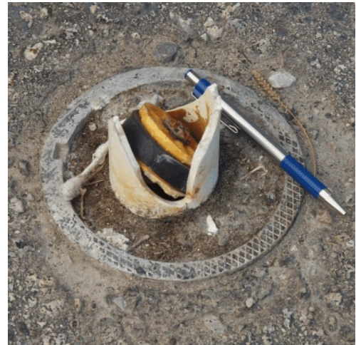
Broken well pipe and a highly ineffective cap. This well was originally installed to test for contaminants on the property. The property is now far more vulnerable because the well wasn't maintained.
