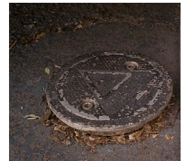
Protective cap flush with ground surface
